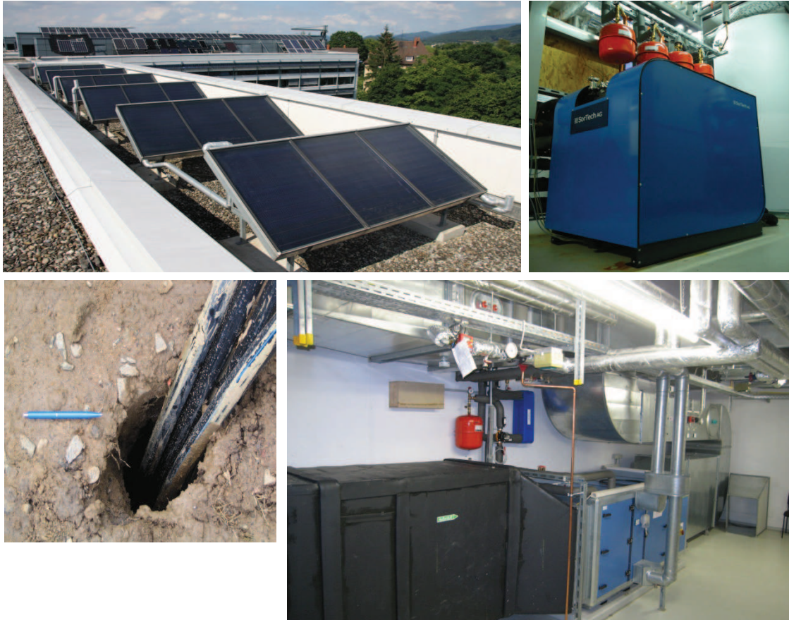
Figure3: Top Left: Flat Collector Area about 22m 2 . Top right: former Adsorption Chiller ACS05. Bottom Left: Borehole with injected pipes. Bottom right: Main Air supply unit of the ISE office department with integrated cold and heating coils
