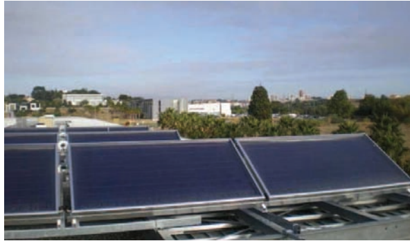
25 m 2 of double glazed solar collector
