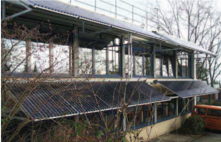
Figure 3: Evacuated tube collector field at the main building of the Technical College Butzbach. Also an effective shading of the rooms can be achieved by the assembly of the collectors. Source: Fraunhofer ISE
