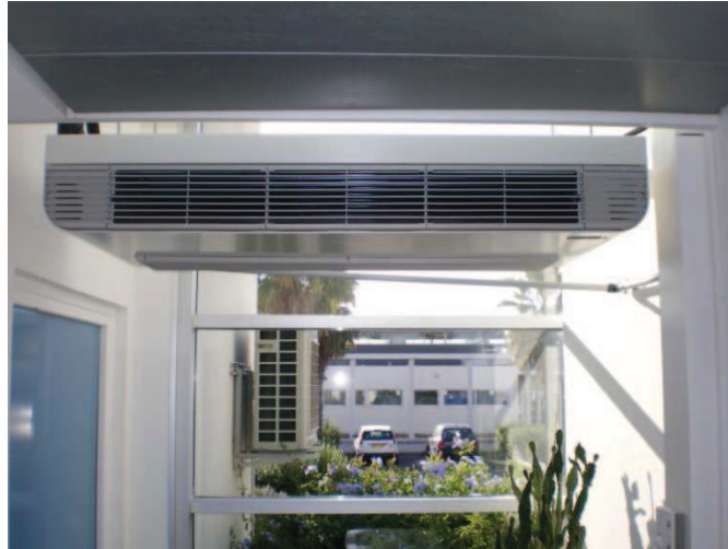
Fan coils for the distribution system
