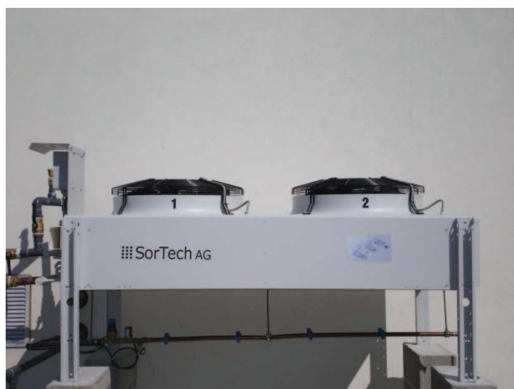
Drycooler used at the perpignan installation
