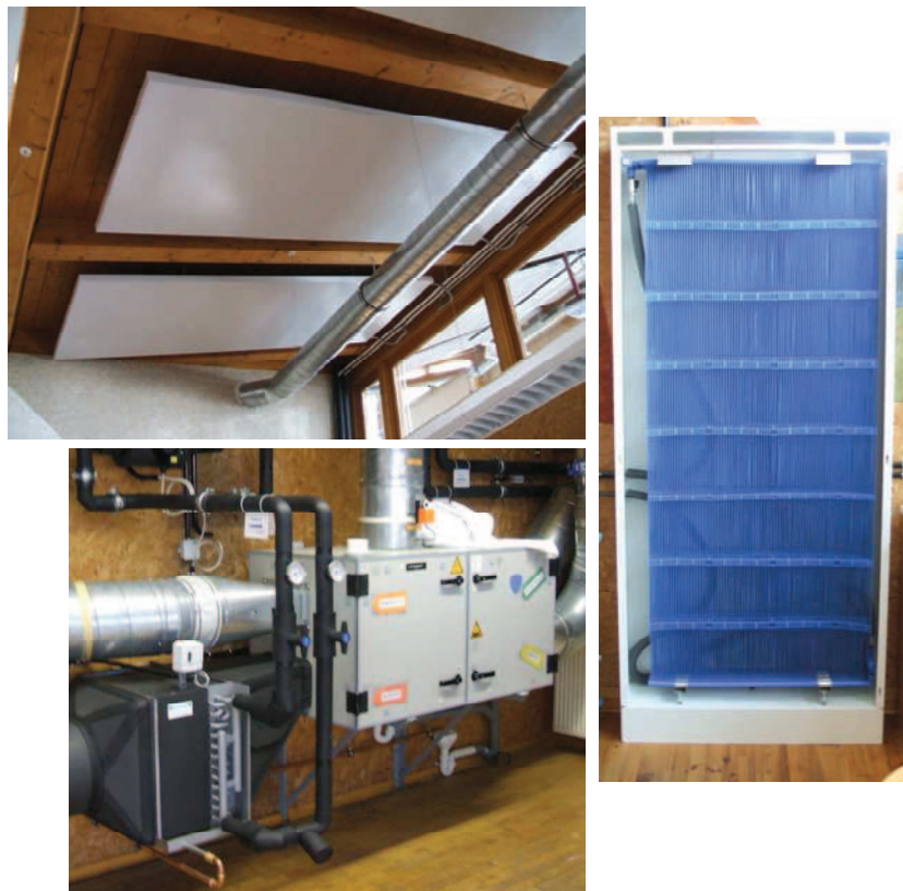
Figure 2: Cold distribution systems in the seminar rooms. Top: chilled ceiling elements; right: cooling shaft (without cover) for silent cooling and air dehumidification. Bottom: one of two air handling units with heat recovery and supply air cooling and dehumidification. The air handling unit in the seminar room was insulated additionally against acoustic noise. Source: Fraunhofer ISE
