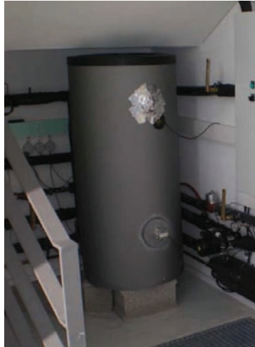
Hot storage tank of 300 liters
