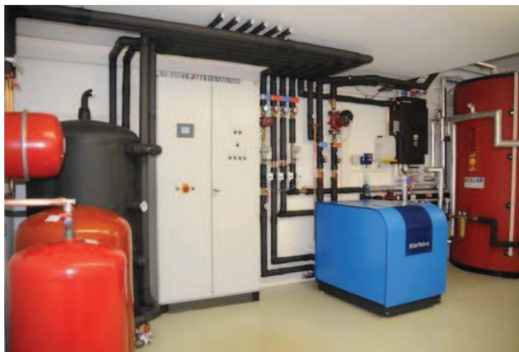
Figure 1: Technical room MA34 solar cooling plant in Vienna (Source: SOLution)
