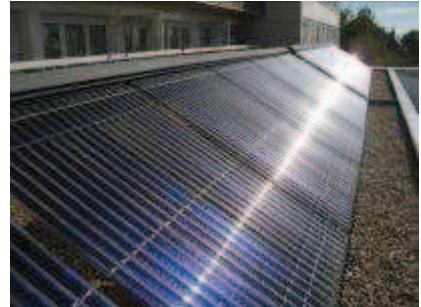
Solar collector field
